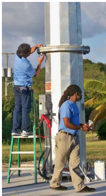
Workers install a 10-kilowatt wind turbine at the St. Croix Reformed Church and Kindshill School in St. Croix. Photo from Don Buchanan, VIEO, NREL 20418
